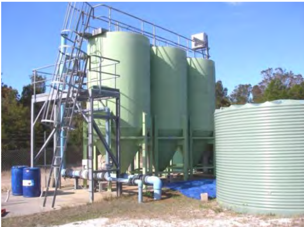
Sand filters at Stuarts Point WTP are used to remove heavy metals and impurities from the source water
