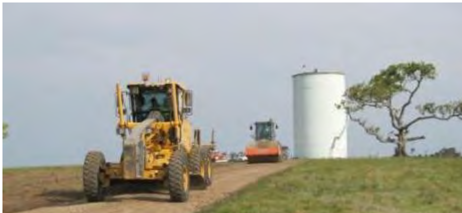
Construction of a new road in 2013 to Clybucca Reservoir has improved access to the site
