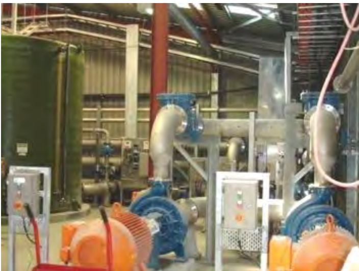
Pumps inside South West Rocks Water Filtration Plant. This plant uses new membrane filtration technology to filter the raw water supply prior to distribution
