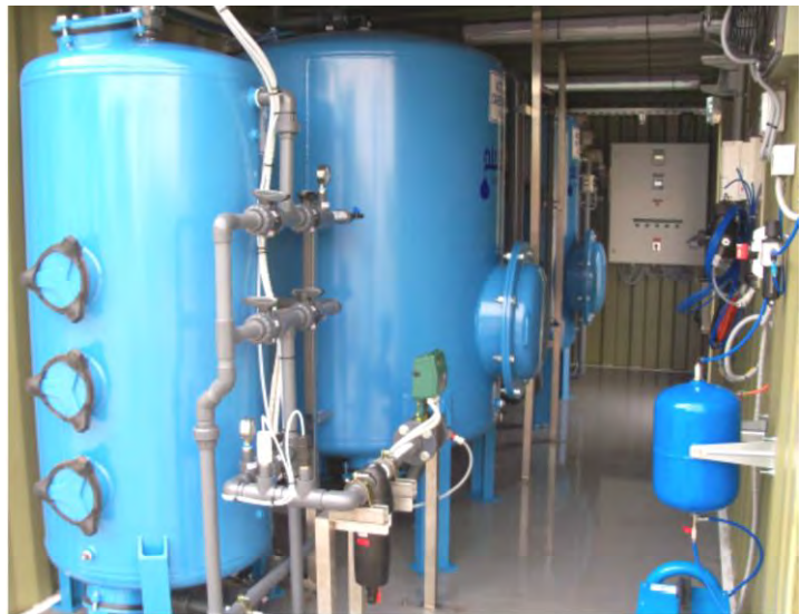
Media Filter tanks inside Bellbrook treatment plant
