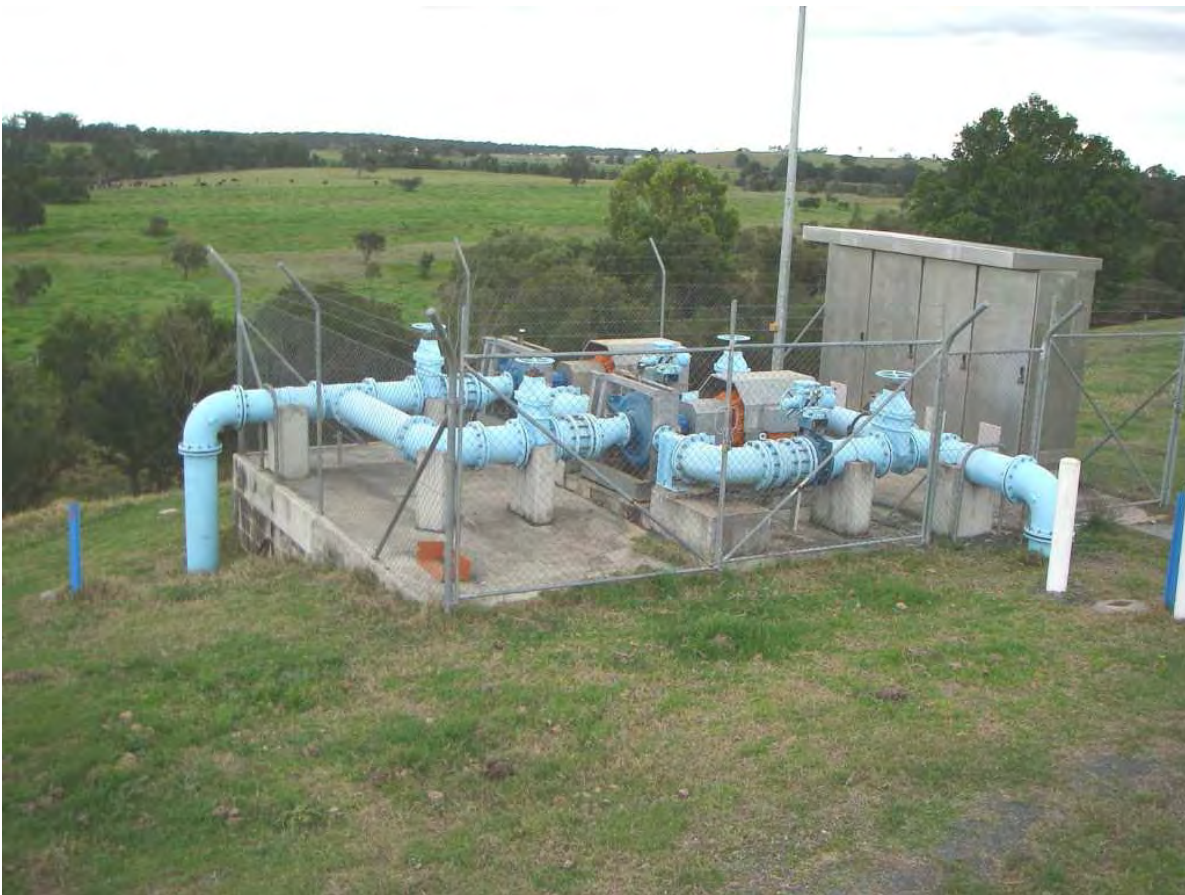
Belgrave Falls Booster Pumping Station
