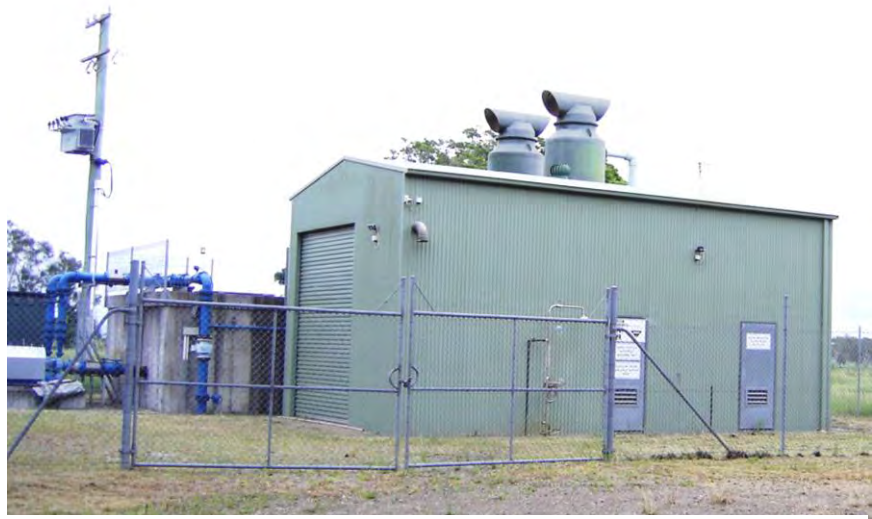
Dosing station at Kinchela which can be utilised as an emergency water system
