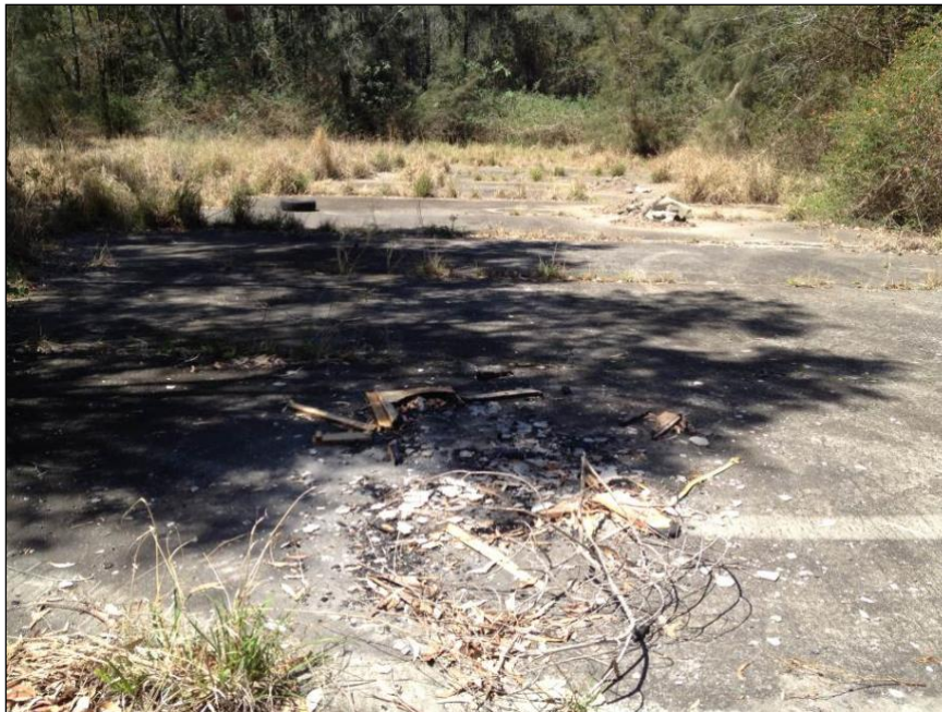
Figure 8. Concrete slab believed to be foundations of former MDL Mineral Separation Plant. Slab location shown as 'B' in Figure 2.
