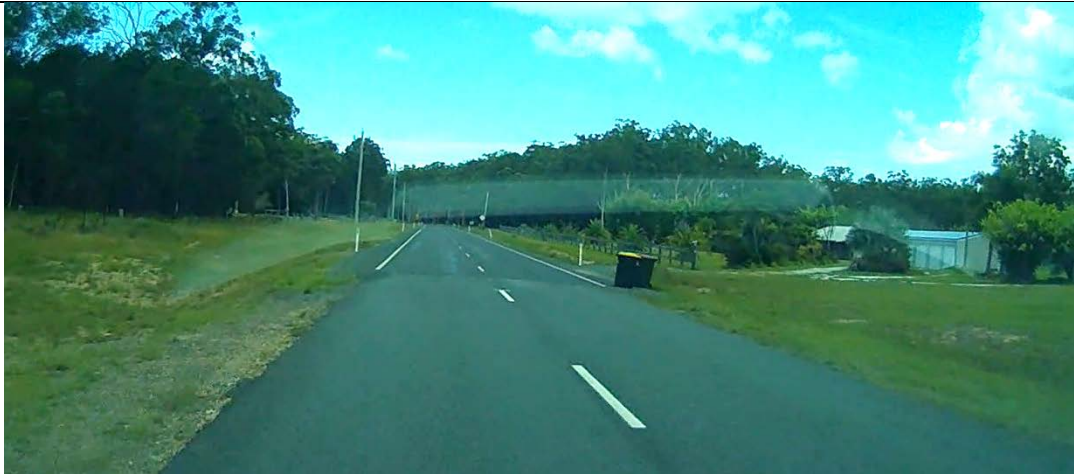
Figure 2.5: Crescent Head Road, showing a join between new and old sections of road
